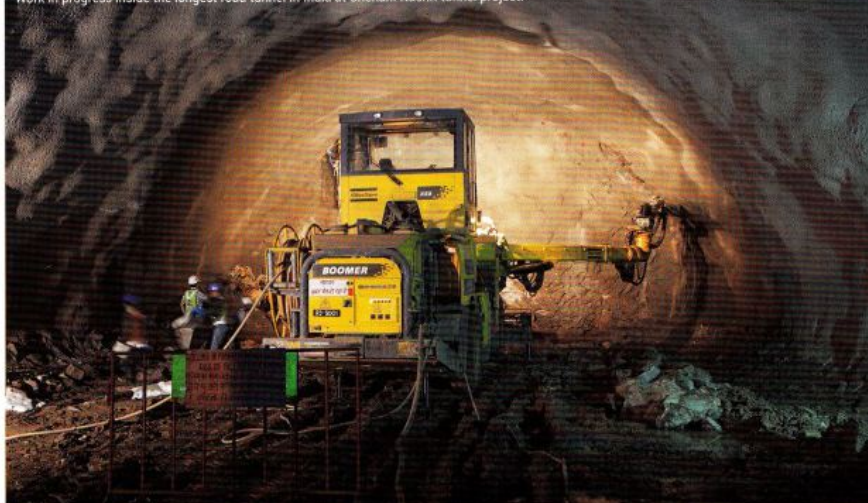
Work in progress inside the longest road tunnel in India at Chenani Nashri tunnel project.
